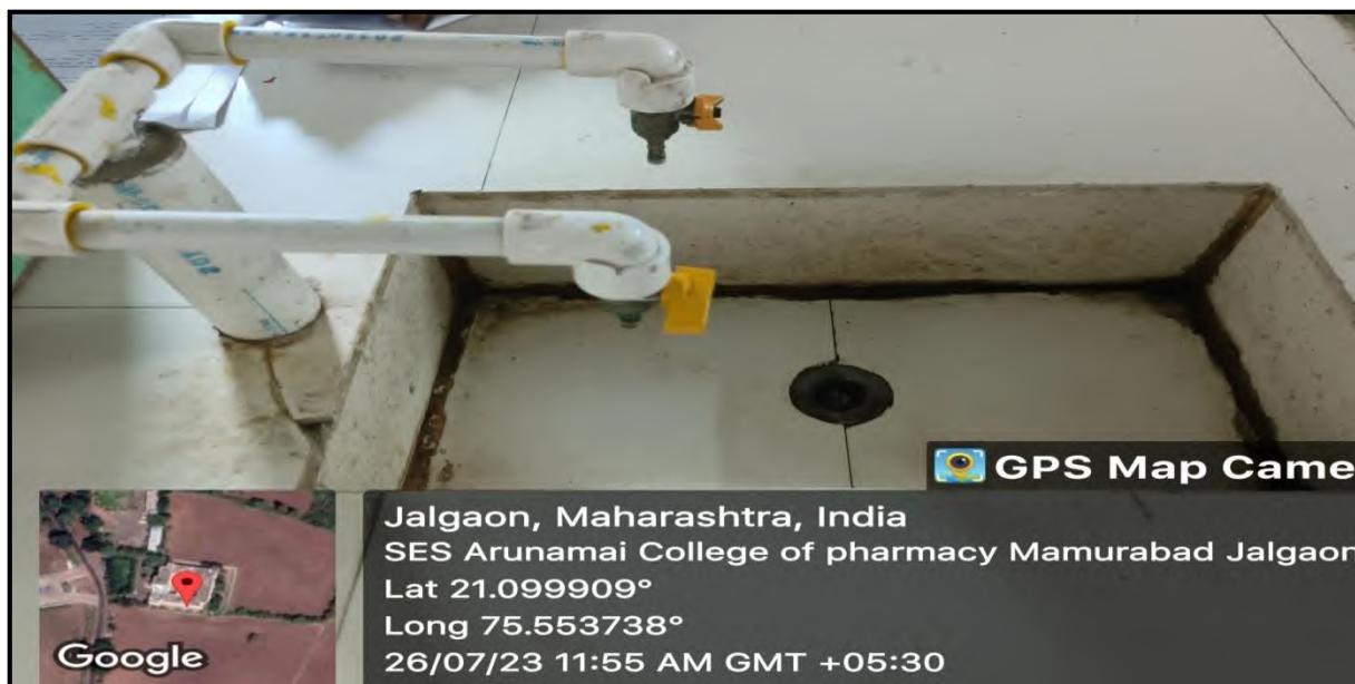
Geotag Image: Water-saving low-flow faucets
