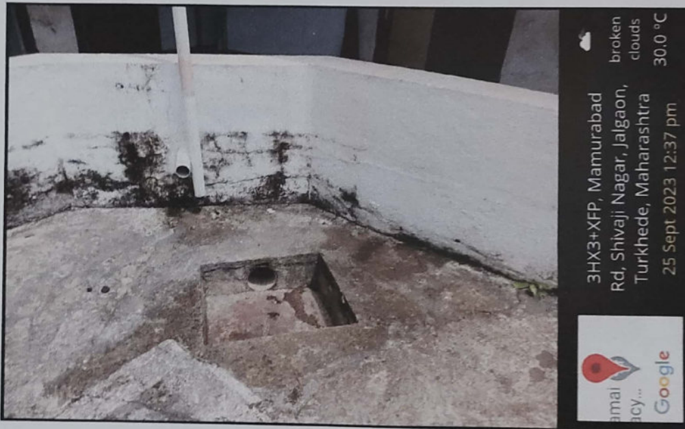
Geotag Image: Inner Water Drainage
